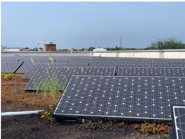
Photovoltaic plant on the roof
